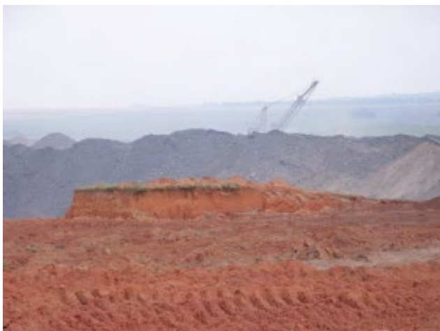
Soil stripping being too close to the mining face
