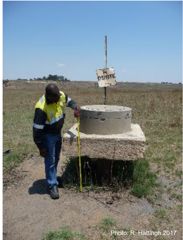
Settlement around a monitoring borehole on dragline-placed spoils
